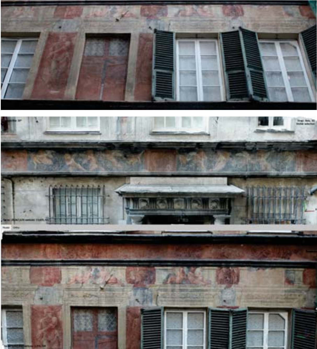
Fig. 4: On the top photographic assessment during the inspection; Detailed orthophoto of the painted decorations in the elevation strip of Piazza Pinelli decorated façades, taken from drone aerophotogrammetry.
