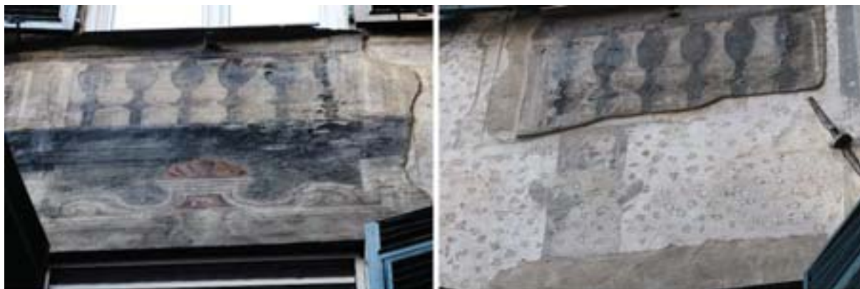
Fig. 2: Stratigraphy of the pictorial decorations of the façade of a building in Piazza Pinelli in Genoa.
