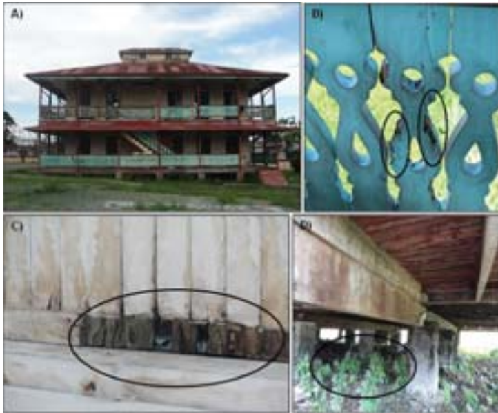
Figure 3. Casa Misionera de la Iglesia Bautista (W - Type 1 - 01). A) Front view. B) Damage caused by insects (termites) (indicated with black circles). C) Damage caused by humidity and fungi (indicated with a black circle). D) Presence of vegetation under the structure (indicated with a black circle).
