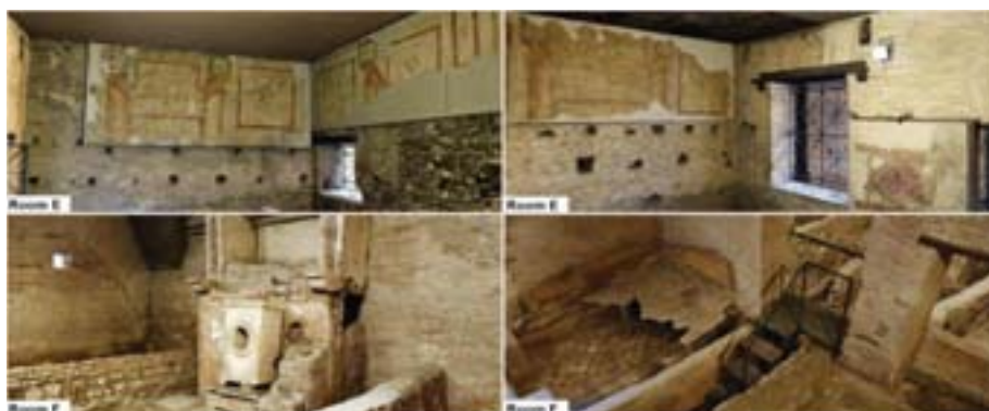
Figure 12B. Rendered images from the 3D model for the target rooms (E on top and F on bottom).
