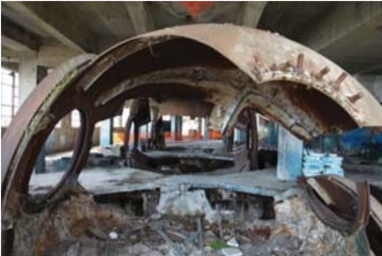
Figure 7. Image taken at elevation of the boilers area (204 meters a.s.l.) (Source: Carlo Vannini).
