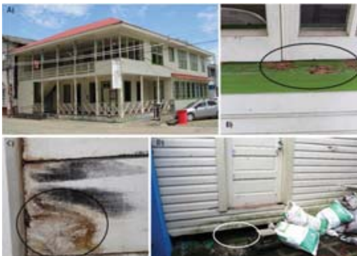
Figure 4. Antigua Capitanía de Puerto (AAA - Type 1 - 01). A) South and East view of the façade; B) Damage caused by insects (termites) (indicated with a black circle); C) Damage caused by humidity and fungi (indicated with a black circle). D) Presence of vegetation under the structure (indicated with a white circle).
