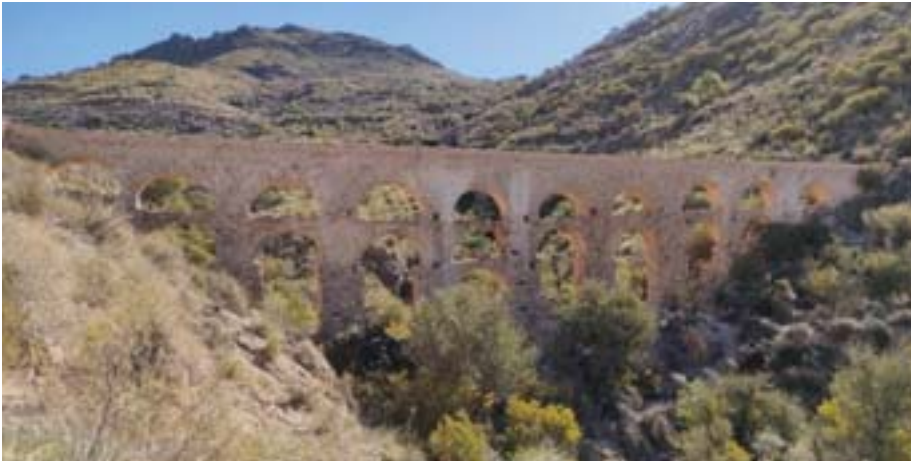
Figure 3. Current conservation state of the aqueduct.
